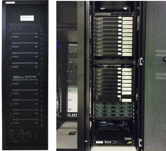
Figure 2.3 Intrinsically Safe DCS Isolation Station Group
